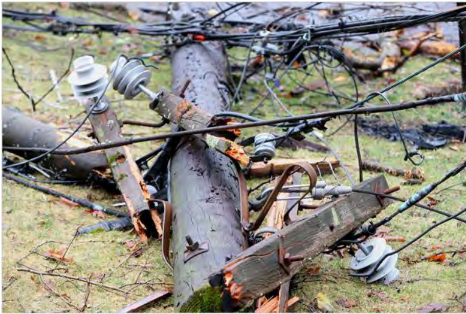
Storm damage in Westchester County, NY, March 12-15, 2010. Source: James Estrin / The New York Times
