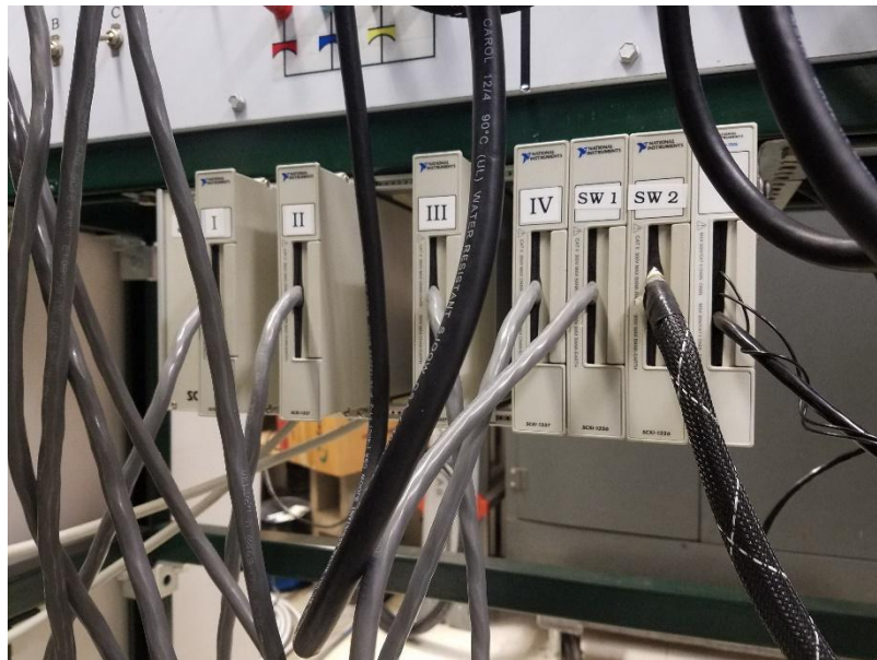
Figure 6. Chassis that holds the four SCBs and two Switch Boards (SW).
