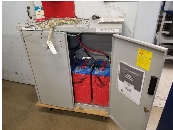
Figure 4. Lithium Ion Battery, located in IPSL
