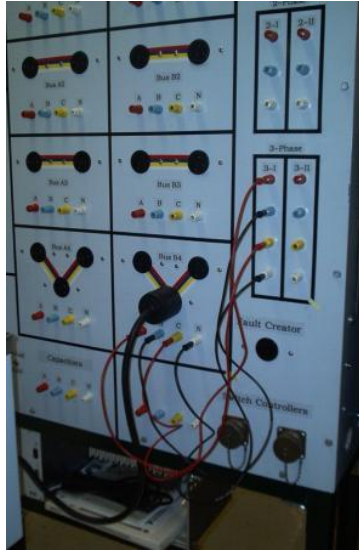
Figure 7. Wiring Connection for a 3-phase Resistive Load (3-I) on Bus B4
