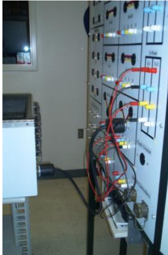
Figure 6. Wiring Connection on Bus B4 Between the Feeder Box and the Transfer Station
