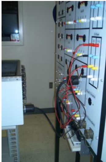
Figure 7. Wiring Connection on Bus B4 Between the Feeder Box and the Transfer Station
