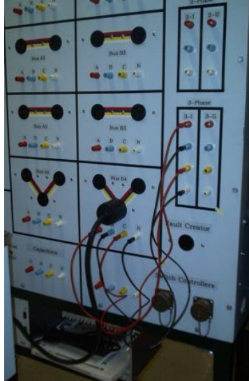
Figure 8. Wiring Connection for a 3-phase Resistive Load (3-I) on Bus B4
