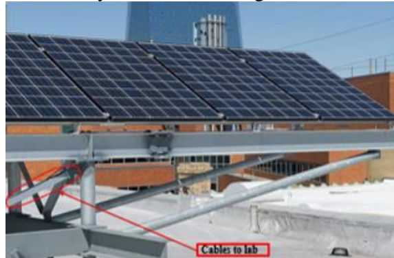
Figure 20: Solar Panels on Main Building
