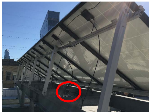
Fig. 3. Master DAQ location beneath array.
