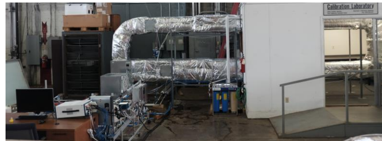
Water-source heat pump
